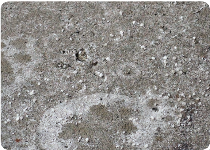
Salt's acidity reacts with highly alkaline concrete to cause damage.
